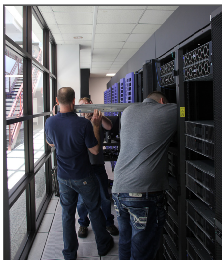
Installation of the Falcon GPU cluster in July 2024.
